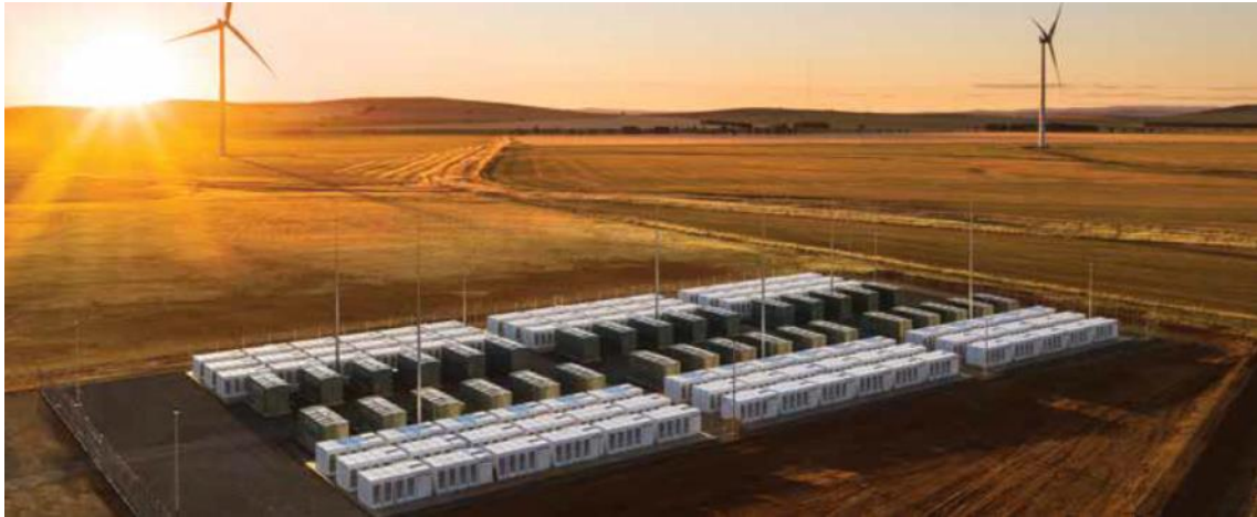
Figure 11. Hornsdale power reserve project in South Australia (Parkinson, 2018).
