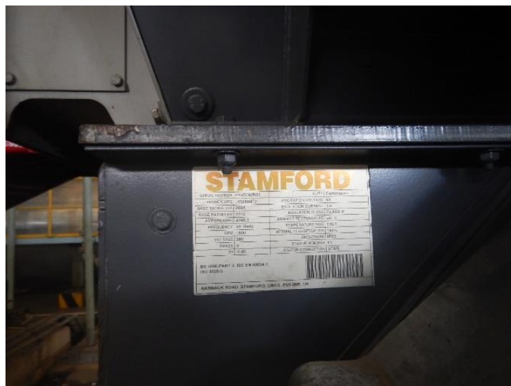
Figure 4. Power Generator Name Plate
